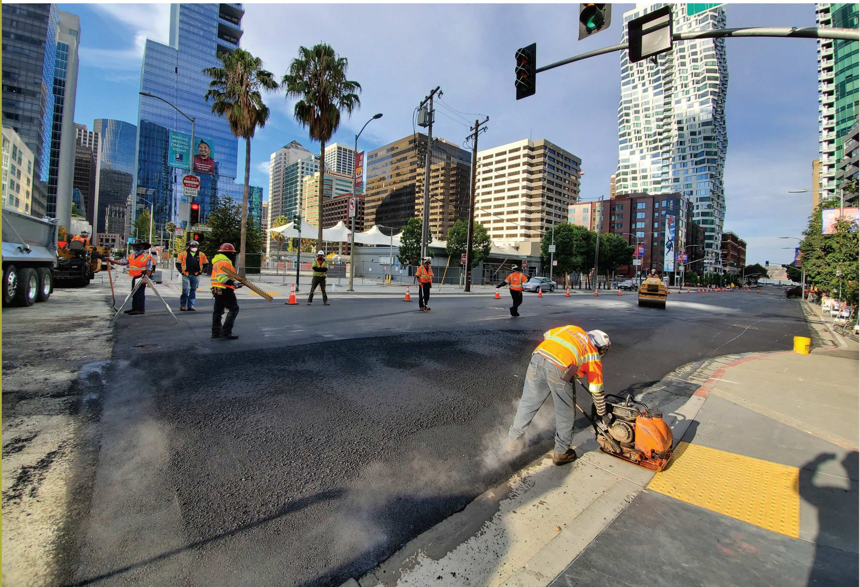
Crews put finishing touches on the new pavement as part of the Transbay Folsom Streetscape Project.
